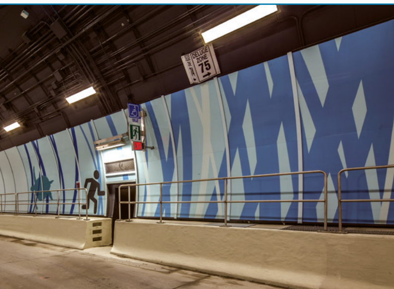
In addition to durability, the Crystal Blue color of the Duranar XL coatings blends well with a series of murals inside the tunnel that depict ocean life.
